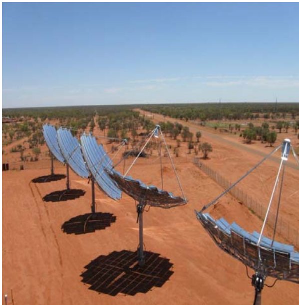
Windorah Solar farm – Queensland’s first 150kW solar farm at the remote south-west Queensland town of Windorah
